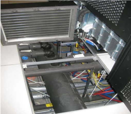
Figure 4. RDHx and Piping
