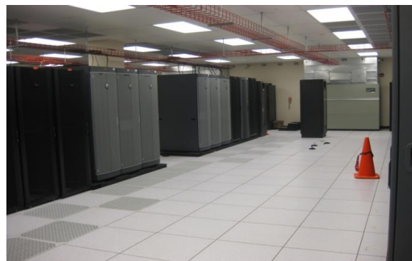
Figure 6. DC2 Lighting, and Perforated Tiles
