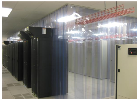
Figure 2. DC1 Hot Aisle Containment
