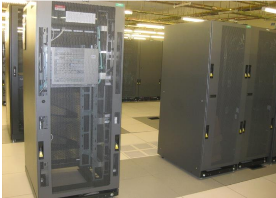
Figure 3. DC3 Openings in Racks
