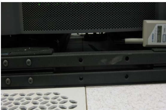
Figure 5. Air Recirculation Under the Racks
