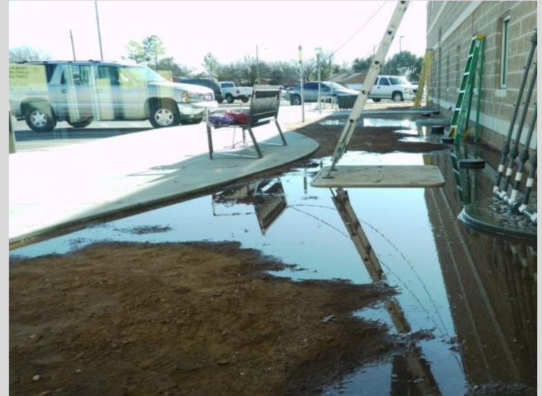
Improper Site Drainage
