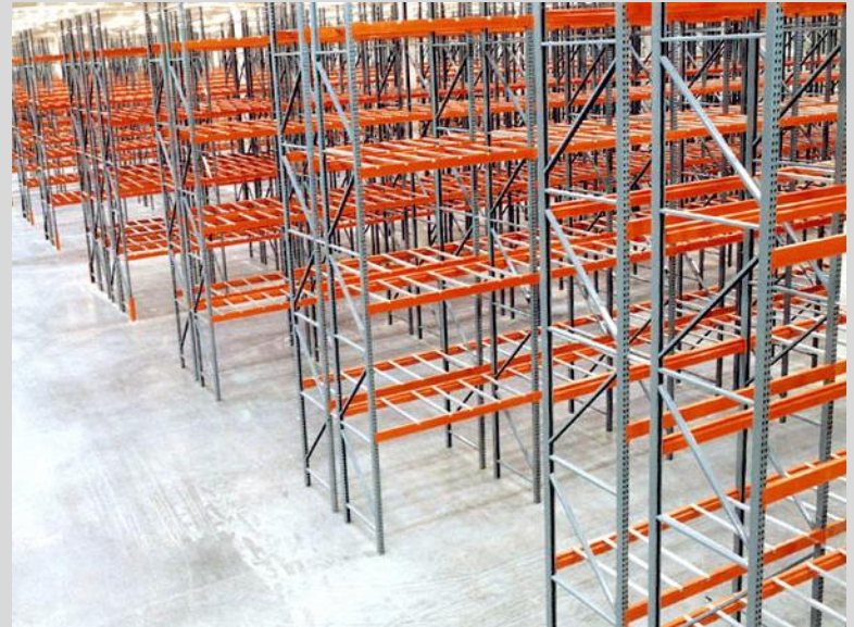
Un-level Warehouse Racking
